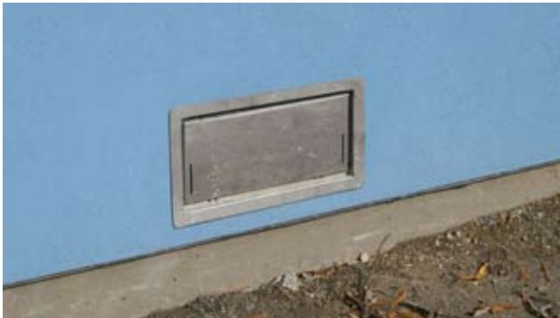
In flood plains, closed crawl spaces have vents in the stem wall, which are designed to pop open under water and then close when the floodwaters recede.
